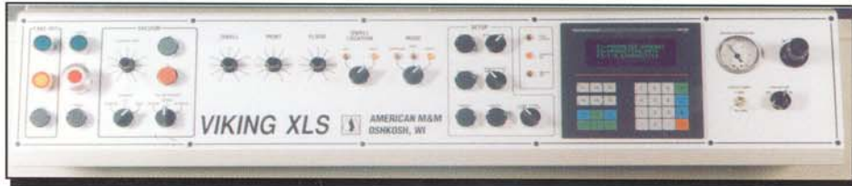
Operator's control panel and air controls
